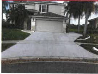
172 HARWOOD CIRCLE Paint/stain
