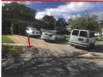
211 WESTMORELAND CIRCLE Pavers on both sides of driveway could not include in photo due to vehicle parking over that area
