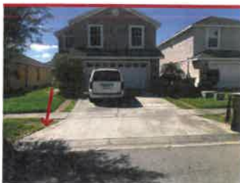
2404 ASHCROFT DR Pavers on side of driveway
